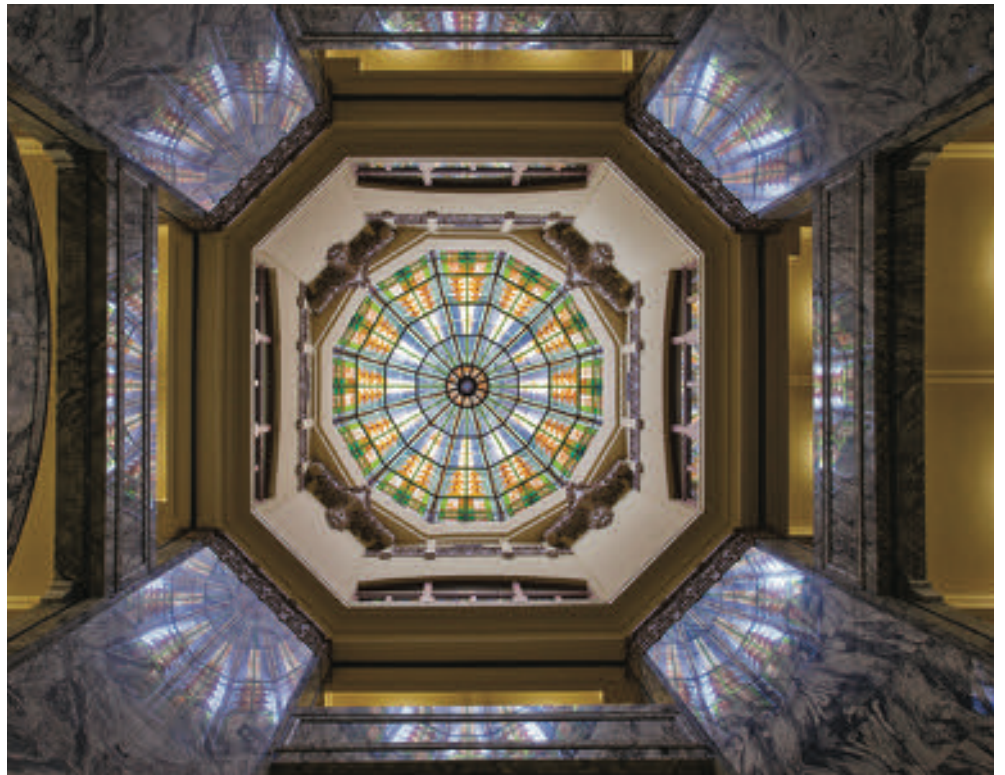
The original art glass under the dome was replaced with a leaded glass piece, its design inspired by floor tiles.
