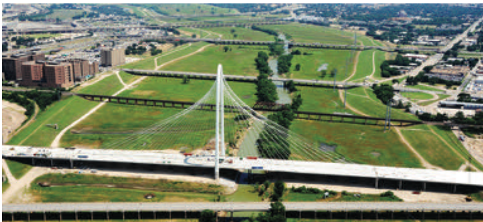
In this view looking south taken in September, construction continued on the Santiago Calatrava-designed Margaret Hunt Hill Bridge spanning 1,250 feet across the Trinity River channel northwest of downtown Dallas.
