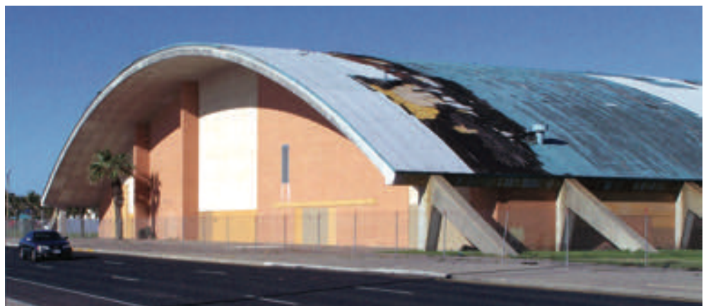
Even as preservationists persisted in efforts to save Corpus Christi Memorial Coliseum, demolition of the downtown landmark began in May. Clearing the site is likely to continue through June.
