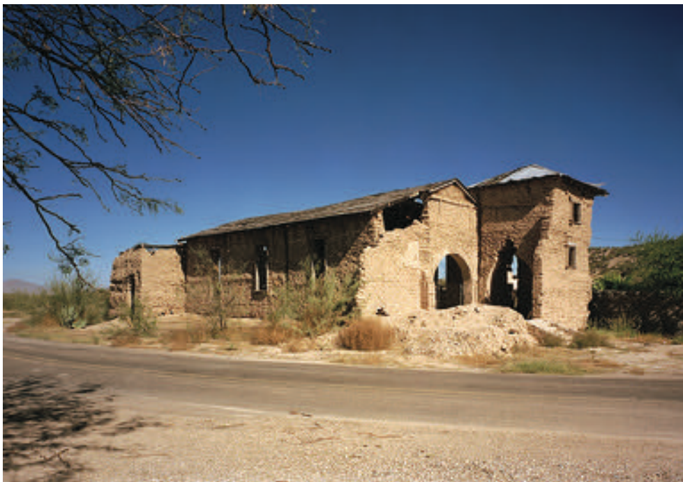
In remote Presidio County, not much is left of the tiny town of Ruidosa except the crumbling adobe walls of the 100-year-old Sacred Heart of Jesus Christ Church. Conservation efforts began last year. Photo by Richard Payne, FAIA.
