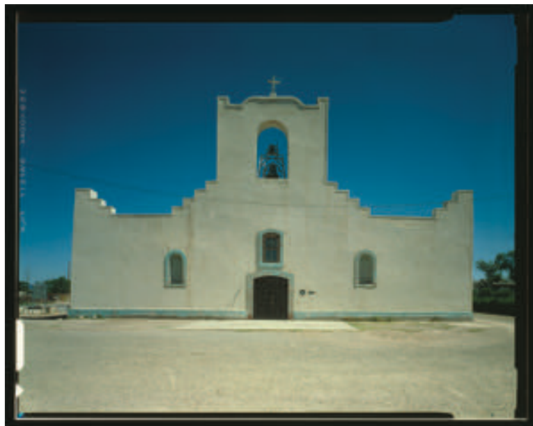
Cracks on the exterior of La Purísima , shown before the recent restoration, developed due to moisture trapped inside the adobe walls. HABS photo taken in July 1980 by David Kaminsky, courtesy Library of Congress, Prints and Photographs Division, Historic American Buildings Survey, Reproduction Number 71-SOCO, 1-23.
