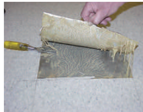
VCT adhesives oozing due to moisture and no vapor retarder under an old school floor. Photo courtesy Howard Kanare of Construction Technology Laboratories.
