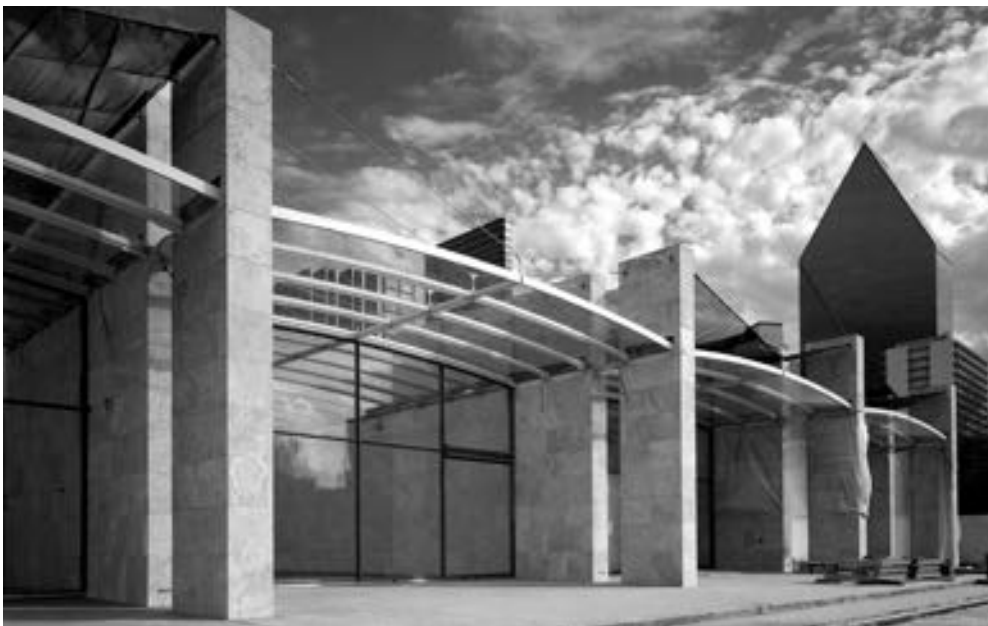
(left) Construction of the Nasher Sculpture Center continued through the summer at the downtown site in the Dallas Arts District. (right) Large works by Mark di Suvero, at top, and Richard Serra are nestled among trees planted in the outdoor sculpture garden; photos by Timothy Hursley.
