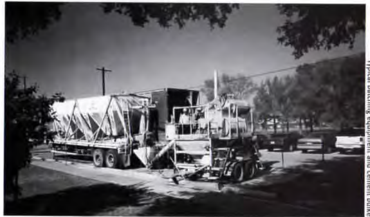
All photos courtesy of Karl Schaeck. Typical batching equipment and cement silo.
