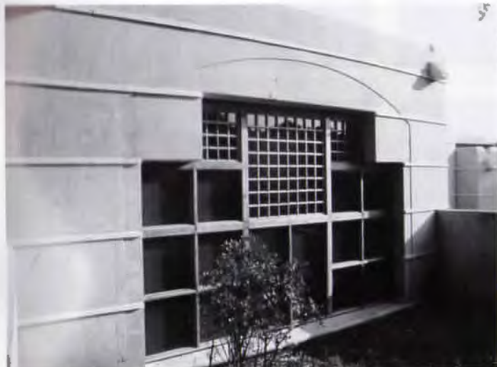
Limestone bands hide concrete tie marks and respond to nearby rock strata.
