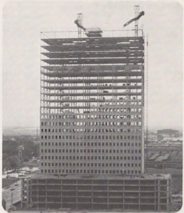
Architect: Christopher Di Stefano & Associates Structural Engineer: Walter P. Moore & Associates, Inc. Contractor: Blount Bros. Corp.
