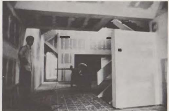
The spaces start to take shape. Gypsum board applied to wood frame work has been taped and floated and is ready for finish and paint.
