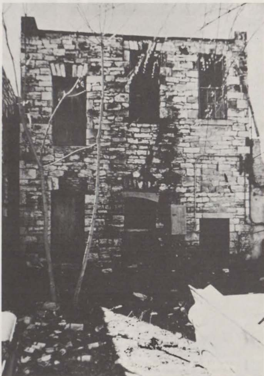
Rear of Building January 1968. Note trash pile, abandoned autos, and rock work that has gathered moss on mortar joints.
