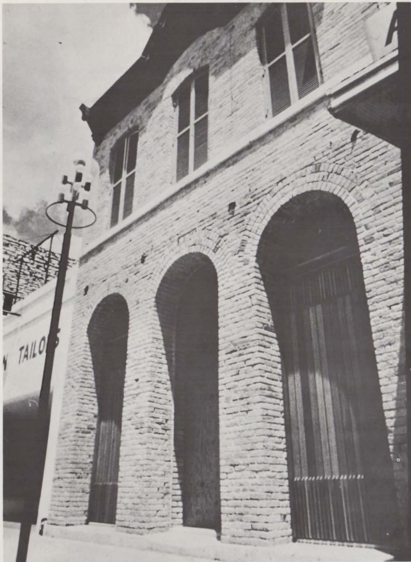
Brick has been sandblasted, mahogany trim and etched glass fill arched openings and even a modern gas light and newly planted tree are in place at the curb side as construction nears completion in December 1968.
