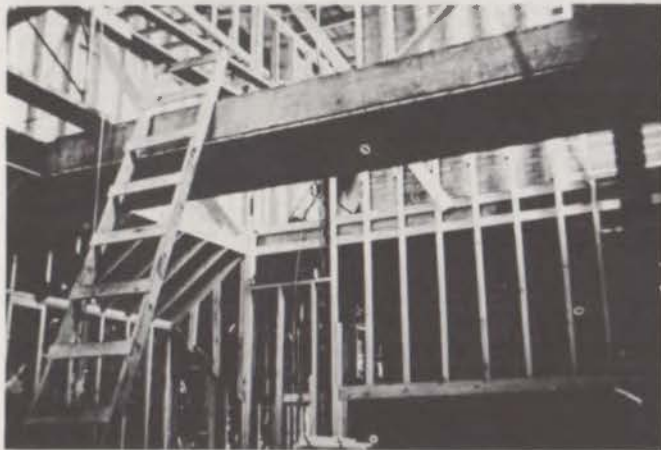
Wood frame work starts to mold interior spaces. Note ladder leaning against portion of existing building, second floor frame work, left in place to become a bridge connecting second floor areas.
