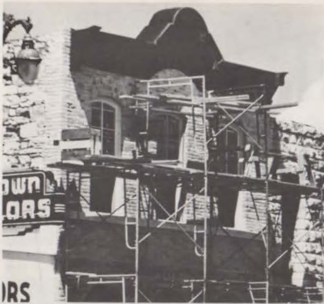
Scaffolding allows sandblasting of brick to remove the dozens of coats of paint that have been applied over the past hundred years.
