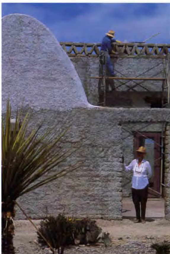
4 Simone Swan stands beside her house near Presidio; the house in Texas is the second adobe project Swan has undertaken.
