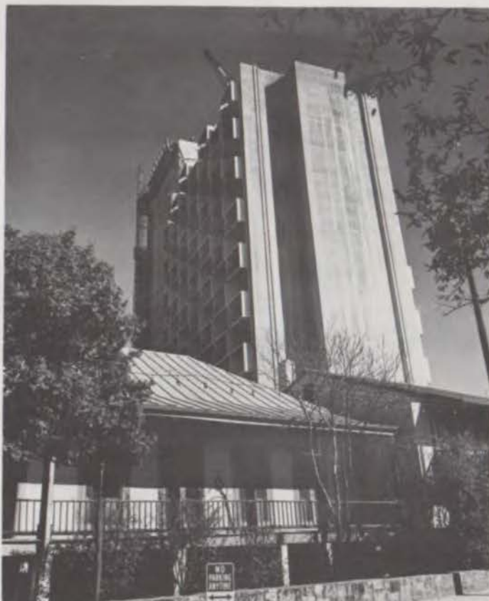
Modular units being placed on south side of elevator core. Due to extremely thin section slip form work on end walls could proceed only a couple of floors above modular units.
