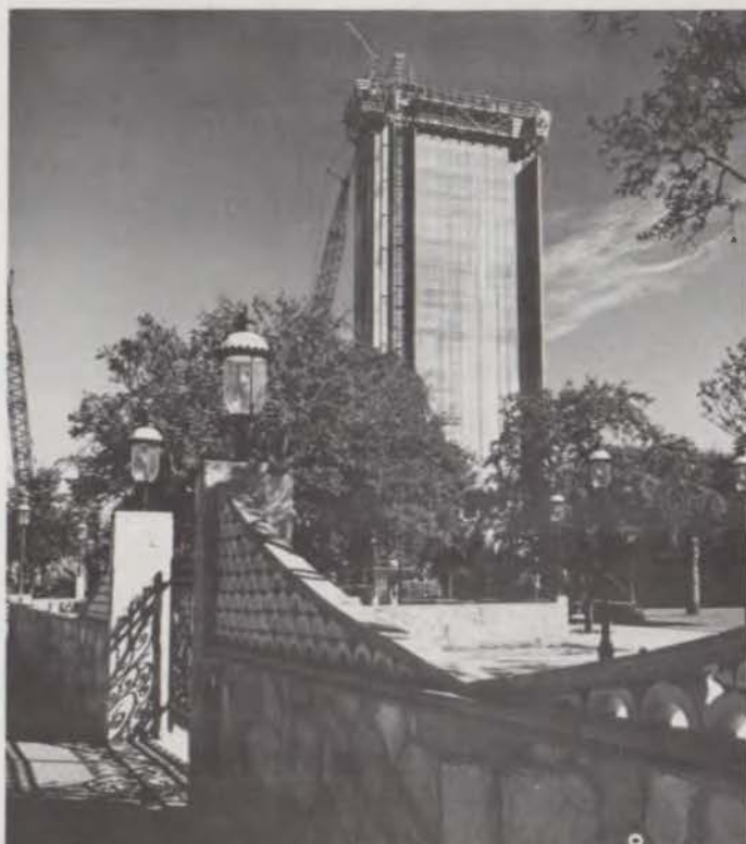
Continuous pouring of concrete into slip form allowed elevator shaft to rise at rate of one foot per hour, around the clock.
