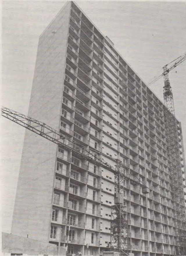
Prefabricated, load-bearing panels of prestressed clay masonry are used for this high rise, frameless building in Southern France.
