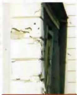
EIFS heavily damaged by high winds in Memphis.
