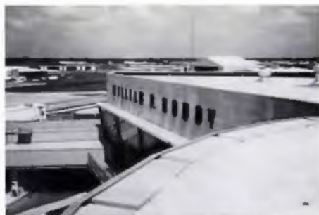
Dow Chemical's Styrofoam Lightguard insulation was used in recent reroofing work at Houston's Hobby Airport, as part of the Dow-pioneered Insulated Roof Membrane Assembly.
