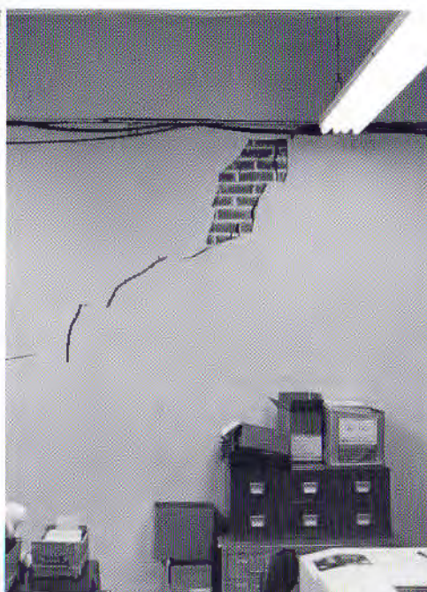
Yawning cracks are starting to show in its walls.
