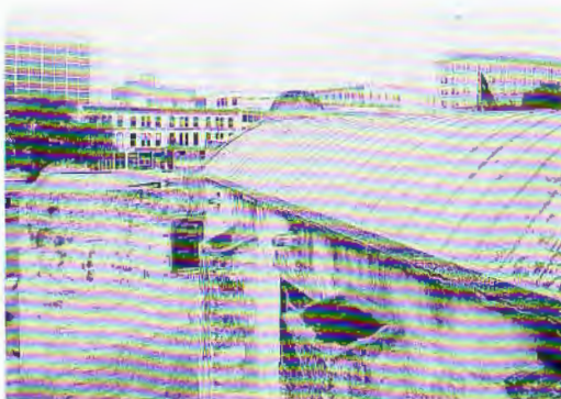
The concrete roof of the Alamo, designed in 1920 by E. Palmer Giles, was clad with lead sheets in 1937 as a Centennial Project.
