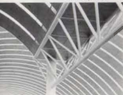
Tubular steel trusses support the series of barrel vaults over the terminal's central block.
