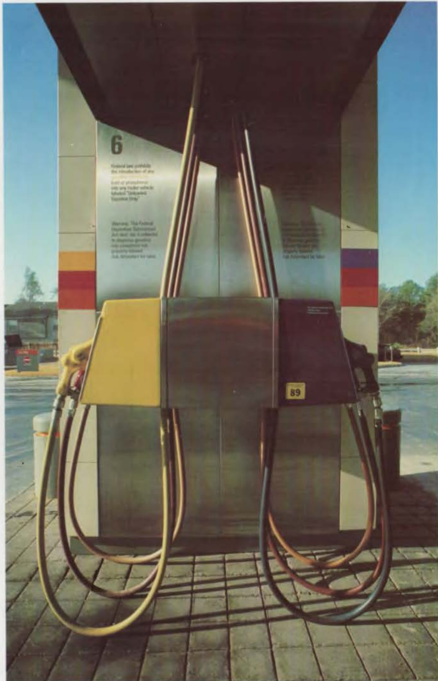
Brightly-colored hoses seem to levitate above curb-less "islands" but are actually connected to high-volume pumps concealed within pylons.
