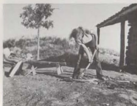
TOP RIGHT: Jowell House on original site near Possum Kingdom Lake, Palo Pinto County. TOP CENTER: Remnants of stone outbuilding with trough for cooling foods at Jowell House. ABOVE: Restoration work in progress on El Capote cabin, log shelter from era of the Republic.
