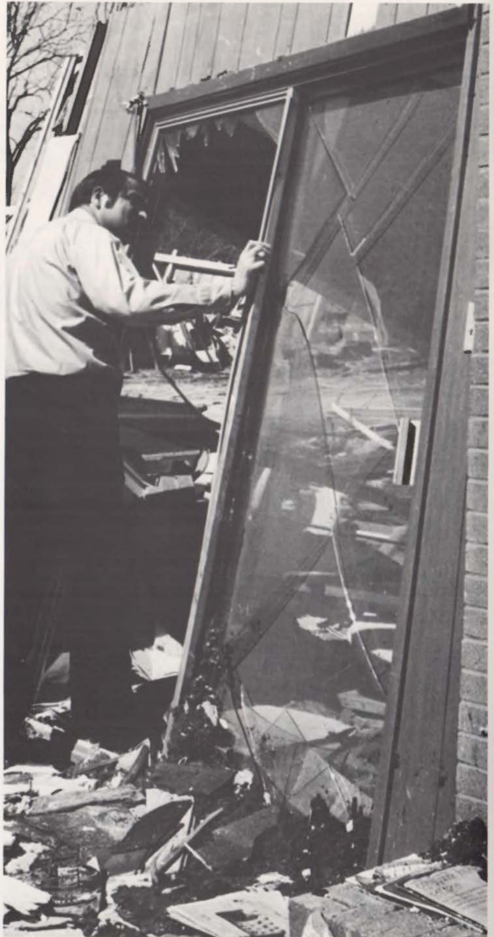
The home of Mrs. Willard Norris was one of many ripped apart by the Burnet tornado. "It was like a freight train," Mrs. Norris recalled. "We're just lucky to be here today." Austin architect Chuck Stahl takes a close look at the structural damage.
