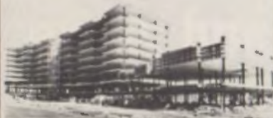
Foxcroft Apartments, Jenkintown, Pennsylvania. Slabs on right being lifted. Others in position. All casting & post-tensioning done at ground level.
