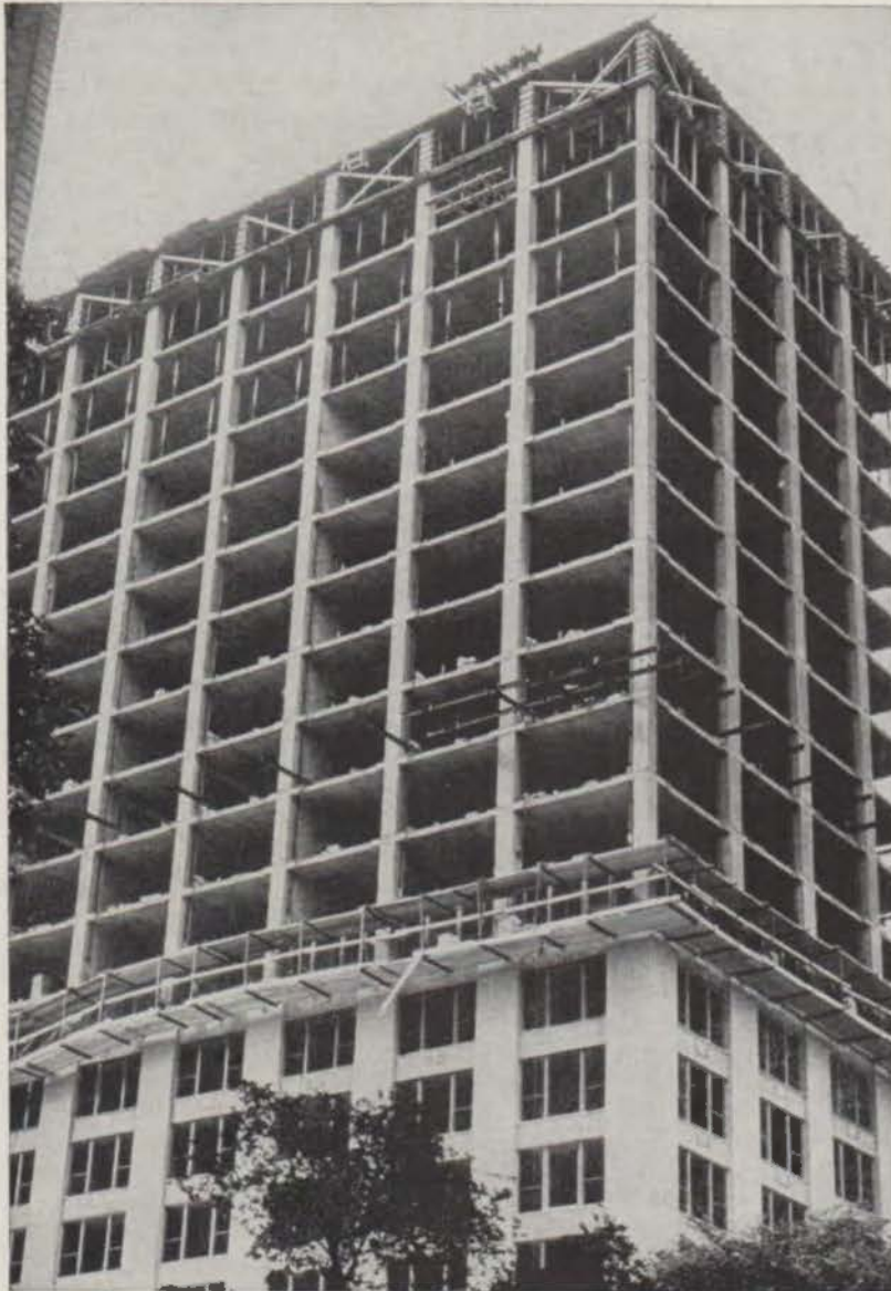
Construction goes fast at 1550 N. Lake Shore Drive. Architects: Shaw, Metz & Dolio, Chicago, Ill. Contractor: Crane Construction Company, Inc., Chicago, Ill.
