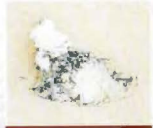
EIFS damaged by hail in Fort Worth.
