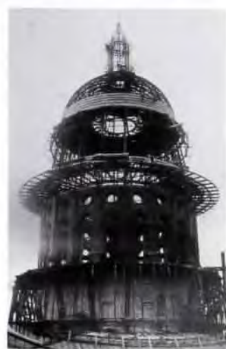
TOP ROW, FACING PAGE AND THIS PAGE: The cornerstone of the Capitol and other period photographs illustrating stages in the Capitol's construction. ABOVE: The iron structure of the Capitol's dome, which, when completed, was a foot taller than the U.S. Capitol in Washington, D.C.
