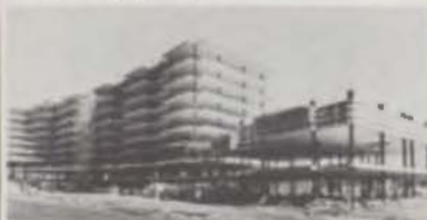
Foxcroft Apartments, Jenkintown, Pennsylvania. Slabs on right being lifted. Others in position. All casting & post-tensioning done at ground level.
