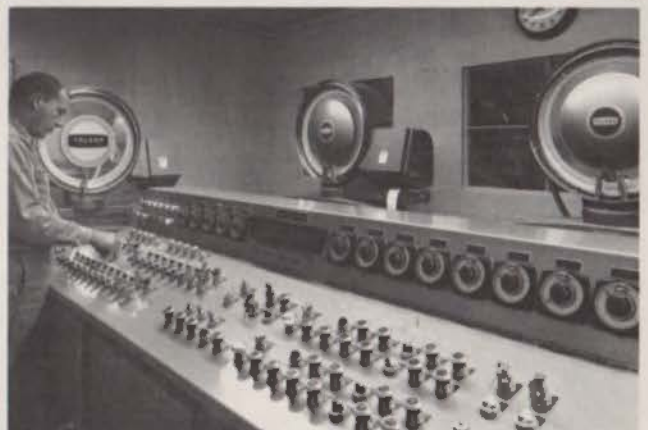
Control panel for automatic batch mixing.
