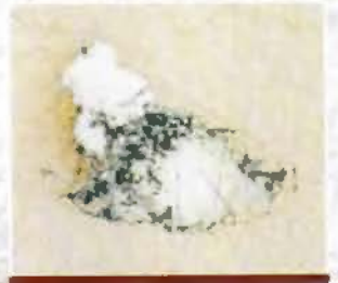
EIFS damaged by hail in Fort Worth.
