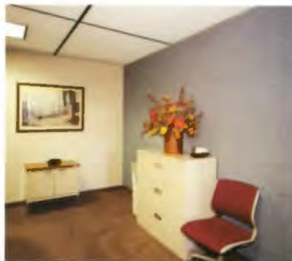
Panels with custom fabric finish appear seamless on renovated office wall.
