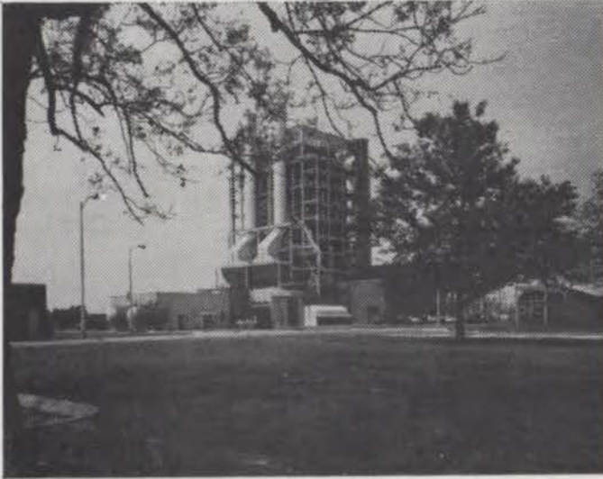
POWER PLANT in New Orleans, Louisiana . . . the electric company's second generating station using 10,000 square feet of Monarch Tile in machine shops, control room and executive offices.
