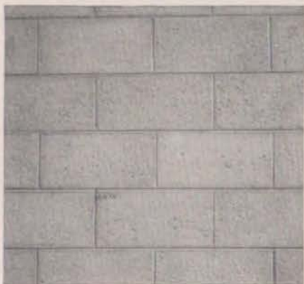
RUNNING BOND. Probably the most widely used pattern of all. Stagger the block in alternate courses so that vertical joints are aligned in every other course. Tool all joints.
