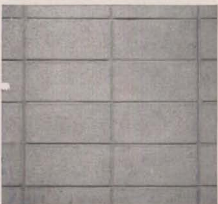
HORIZONTAL STACKING. For interior non-bearing walls this treatment is striking. Place the block in the normal manner but align all vertical and horizontal joints and tool them.
