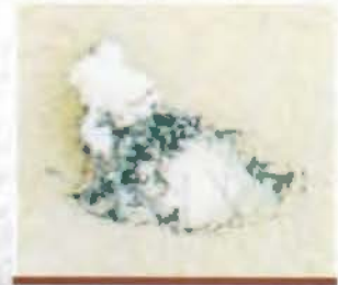
EIFS damaged by hail in Fort Worth.
