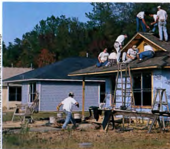
Client: Houston Habitat for Humanity; architect: Gerald Moorhead, FAIA; planner: Tim Hanson, ASLA
