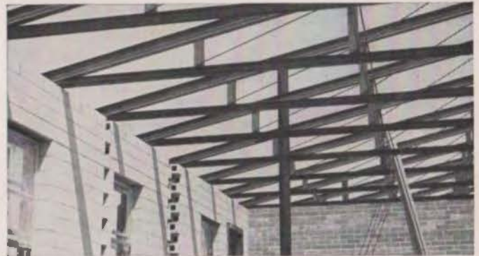
Stran-Steel trusses form clear-span roof over load-bearing masonry walls. Collateral material can be nailed to the steel!
