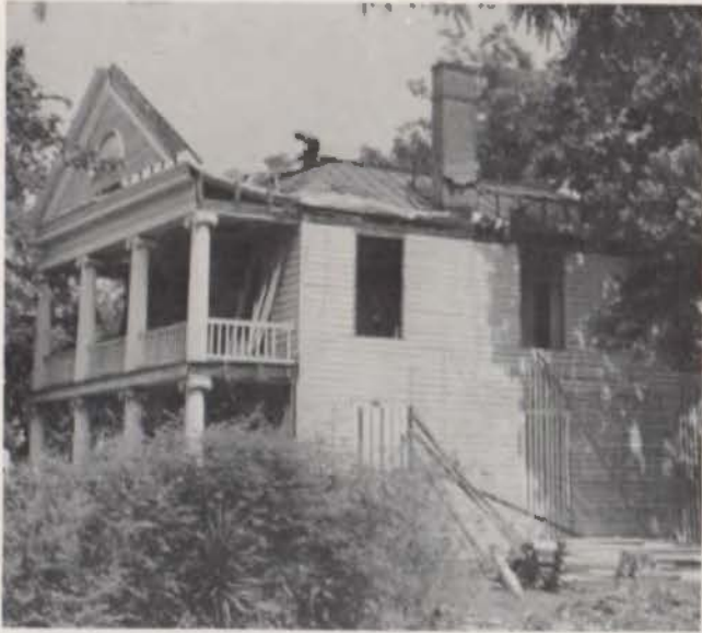
Dismantling uncovered original terne roof and widow's walk, hidden by high gabled roof for many years.
