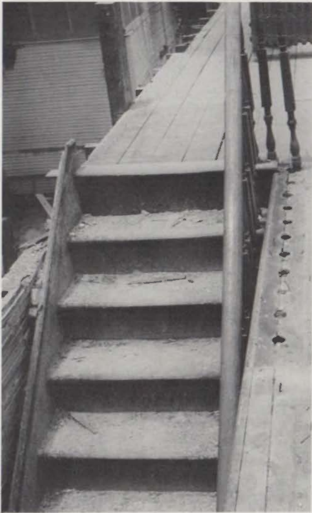
Original stair with the old flooring exposed showed the location and extent of the balustrade.
