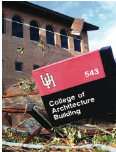
UH's College of Architecture building sustained major roof damage during Hurricane Ike.
