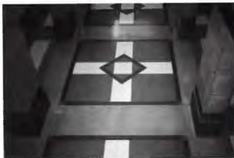
Terrazzo, Texas State Capitol Expansion in Austin, designed by 3D/International, Inc., Houston; Ford, Powell & Carson, Inc., San Antonio, in joint venture.
