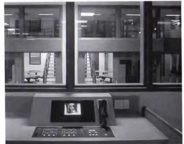
Above: A central monitoring station, with electronic equipment, allows surveillance of jail cells and dayrooms from a single point.
